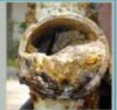
Sewer Pipe Clogged with grease
