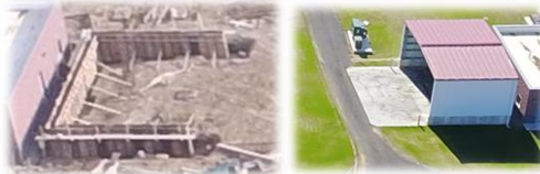
Sludge Storage Building (Cake Pad)
