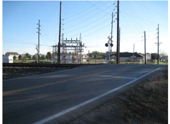
Photo 8: Electrical substation northeast of Site, across Ohio Route 752.
