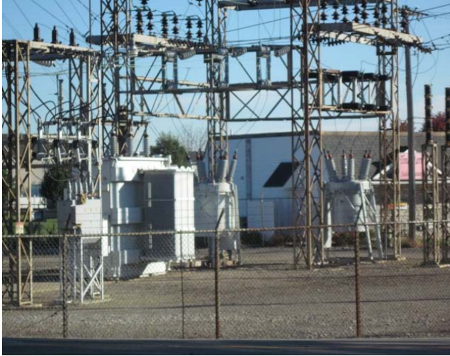
Photo 13: Close up view of substation. Viewing NE.
